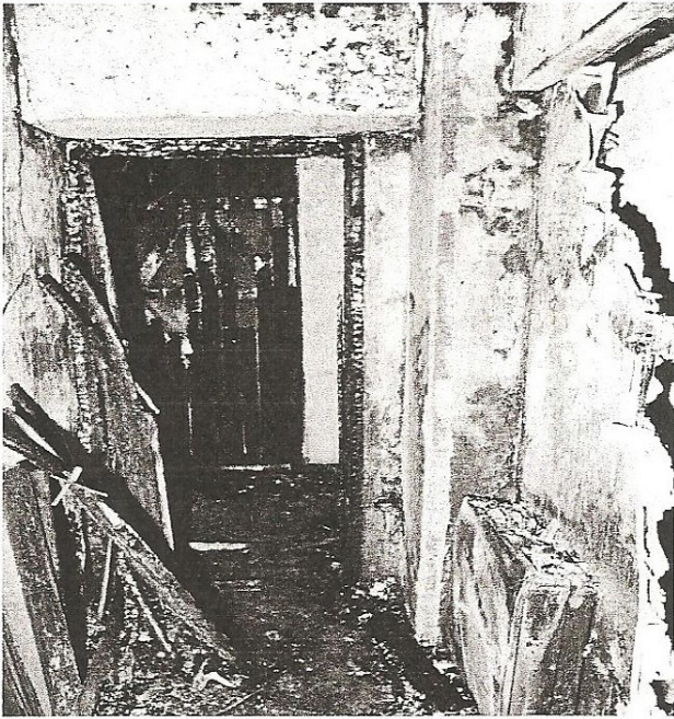
Figure 4 presents a view of the fire scene and indicates the degree of involvement.
